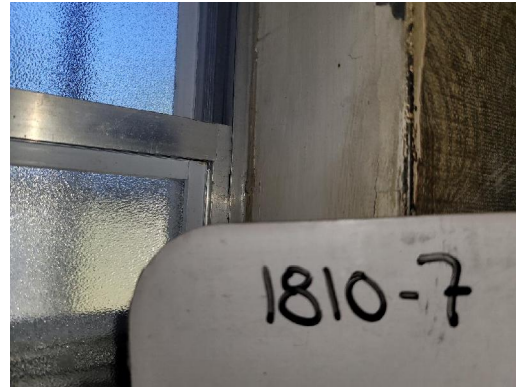
1810-7 Caulk/Tan/White Typical Interior Windows
